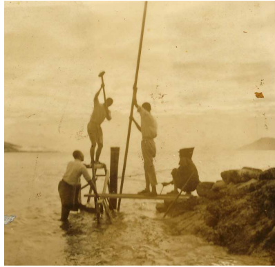
圖片(9)：昔日建築碼頭時的情形，神父修士們充當「洑水銅人」。 The construction of the pier in early days. The Trappists acted as “diving man”.
