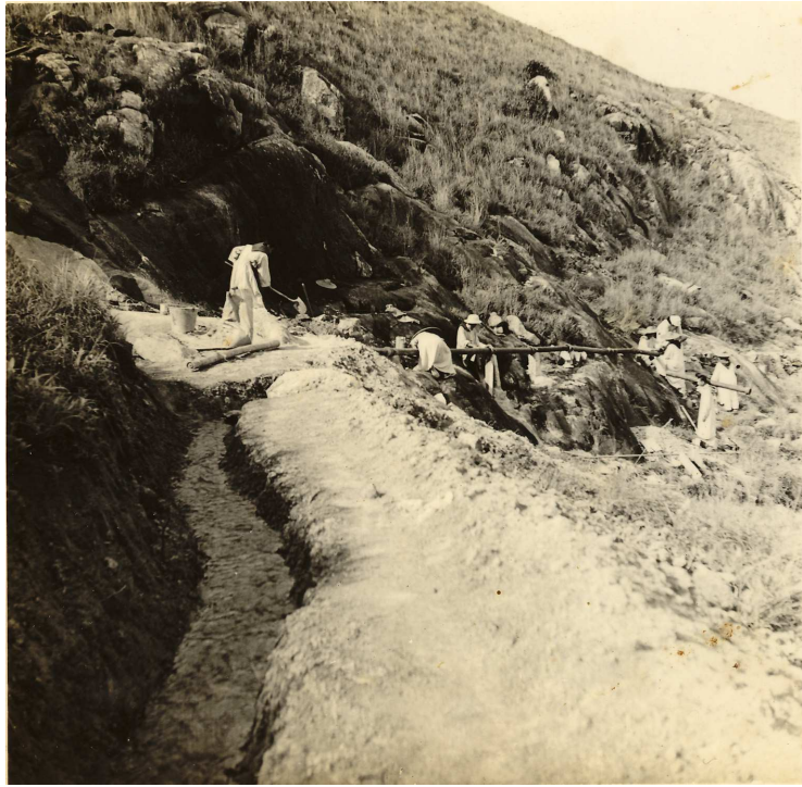
圖片(15)：修士們不畏勞苦在接駁水管，親力親為。 The Trappists are connecting water pipes. They do everything all by themselves.
