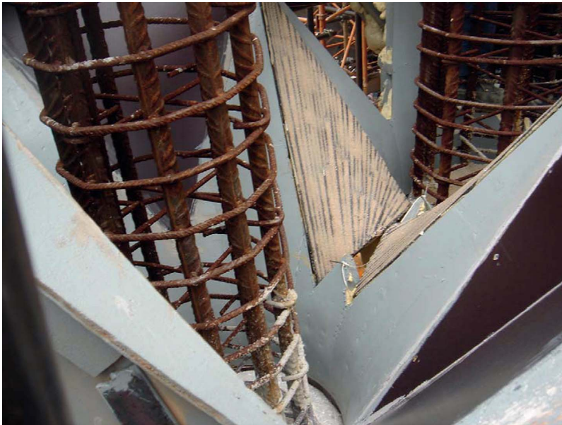
Figure 16. Photographs showing smaller paraboloids that are previously prefabricated (figure is provided in color online).
