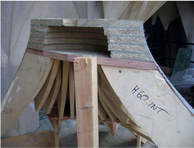
Figure 18. Photographs showing the formwork of the hyperboloids when they are placed on the bottom part of the capital (figure is provided in color online).
