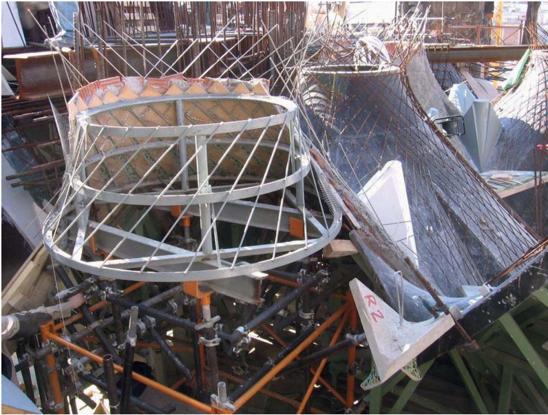
Figure 12. Photograph of a stainless steel soldered net during placement as a frame for the hyperboloids (figure is provided in color online).
