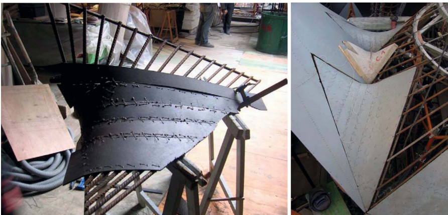
Figure 14. Photograph of the formwork adaptation of its shape to that of the paraboloid's curve (figure is provided in color online).
